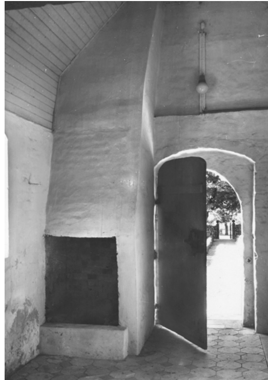
Fig. 12. A fireplace built with bricks in the porch of the church in Sdr. Hygum in southern Jutland. Pieces of molten lead have been found in it. Photo: Elna Møller 1952, the National Museum.
