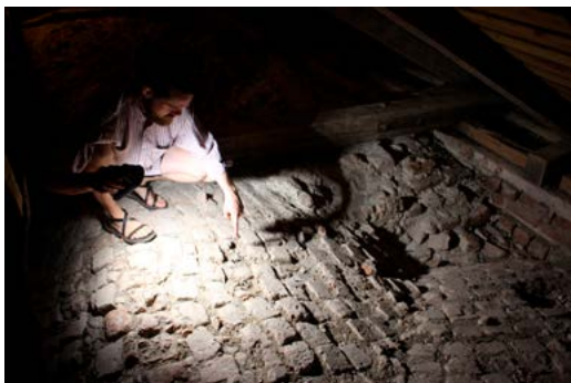
Fig. 5. The area on top of the vaults in the eastern end of the northern aisle where lead drops were discovered and later removed. Photo: Thomas Bertelsen 2018.
