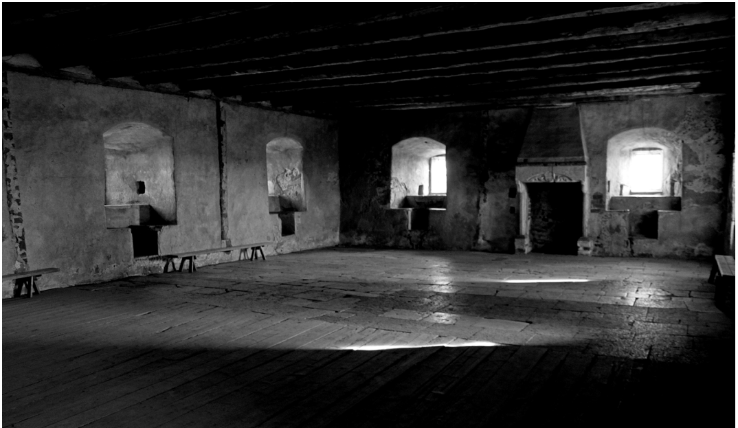
Fig. 6. Room 1 (301) photographed from the western part of the room. Notice the fireplace and the vertical stripes of mortar and bricks. Photo by S. Lind 2012.
