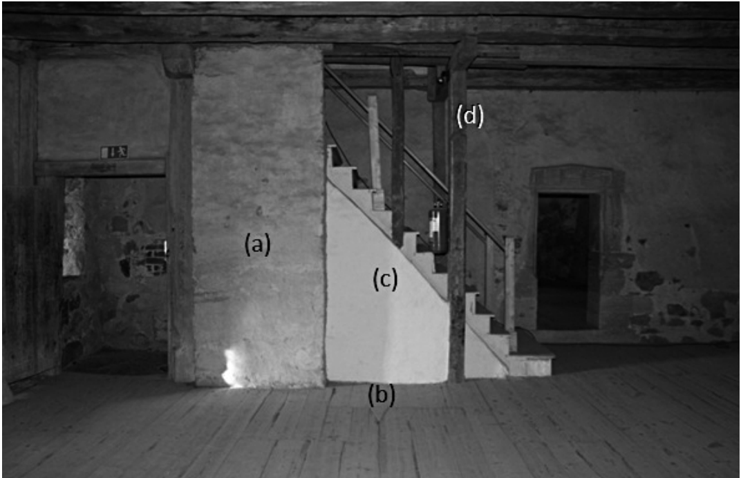
Fig. 10. The staircase photographed from the eastern part of Room 1 (301). The chimney has continued up through the floor just north of the supporting pilaster (a) – a square in the wooden floor (b) can be seen where it once went up. Notice the new plaster and stairs (c) leading up to Room 2 (401), and the remains of the supporting wooden structure (d) at the base of the stairs. Photo by S. Lind 2012.
