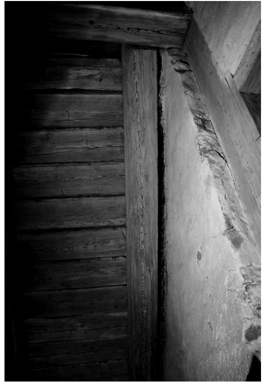
Fig. 11. The stairs leading from Room 1 (301) to Room 2 (401) photographed from underneath, the plaster of the supporting pilaster not reaching up under the supporting beams in the stairway. Notice the substantial beam which the staircase rests upon at its upper end, and how it is joined with the half-timber structure above the doorway. Photo by T. Westergren 2011.
