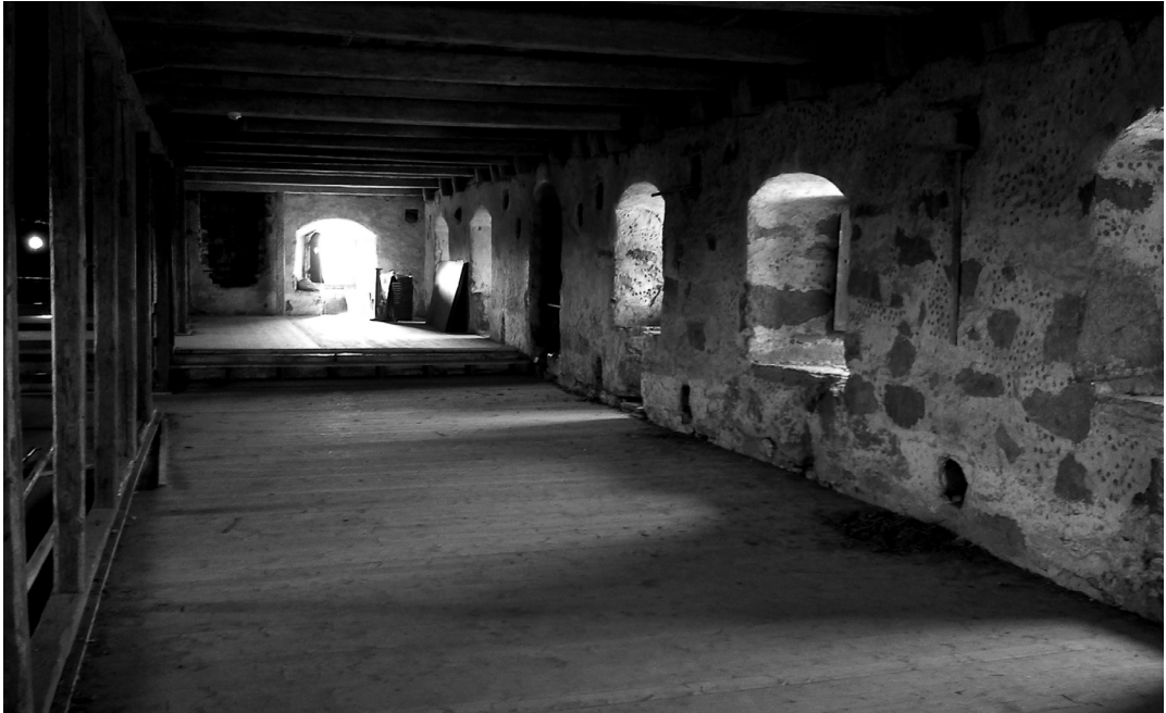
Fig. 12. Room 2 (401) photographed from the eastern part of the room, showing the northern half of “the Archers’ Loft”. Notice the holes between the windows, placed in pairs, and the posts of the truss ending with a faced side, a little beneath the top of the wall – the beams going across the ceiling lying loose on top of the wall and supporting the secondarily built attic. Photo by S. Lind 2010.
