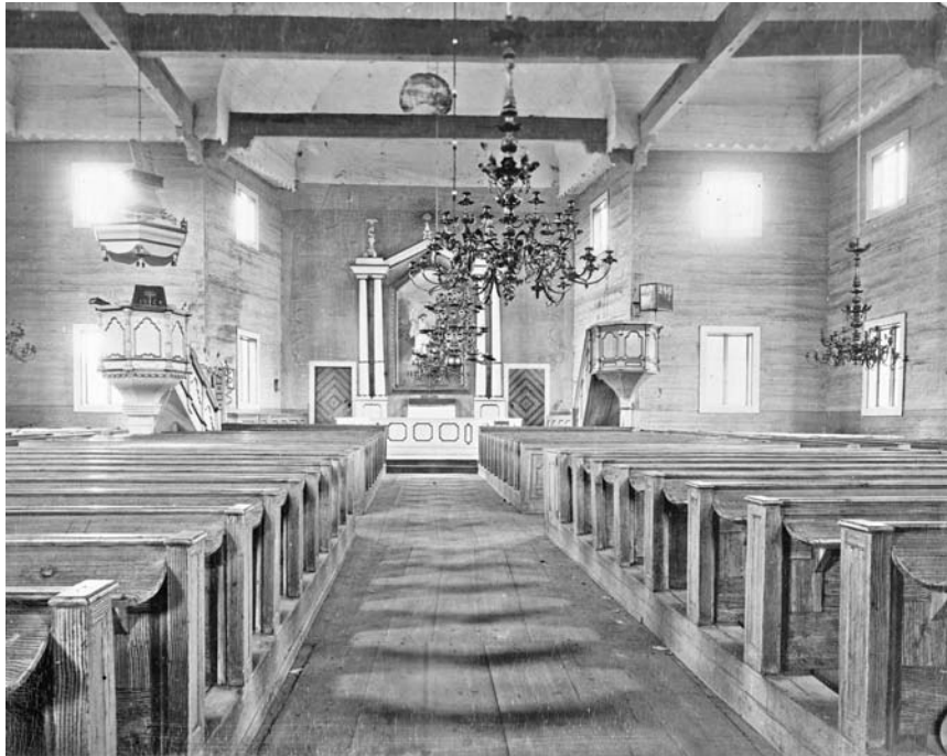
Fig. 6. Interior of Valkeala Church. The tie-beam crossings lack vertical supports. Photo Christian Ganderup 1898. National Board of Antiquities, Picture archives, 3976.
